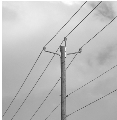
(a) Three-phase 34.5-kV armless construction with covered wire.
